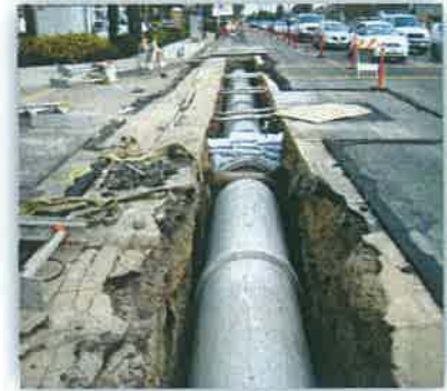
Ball/Bloomfield Storm Drain City of Los Alamitos
