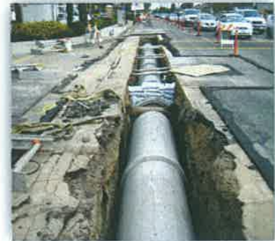
Ball/Bloomfield Storm Drain City of Los Alamitos
